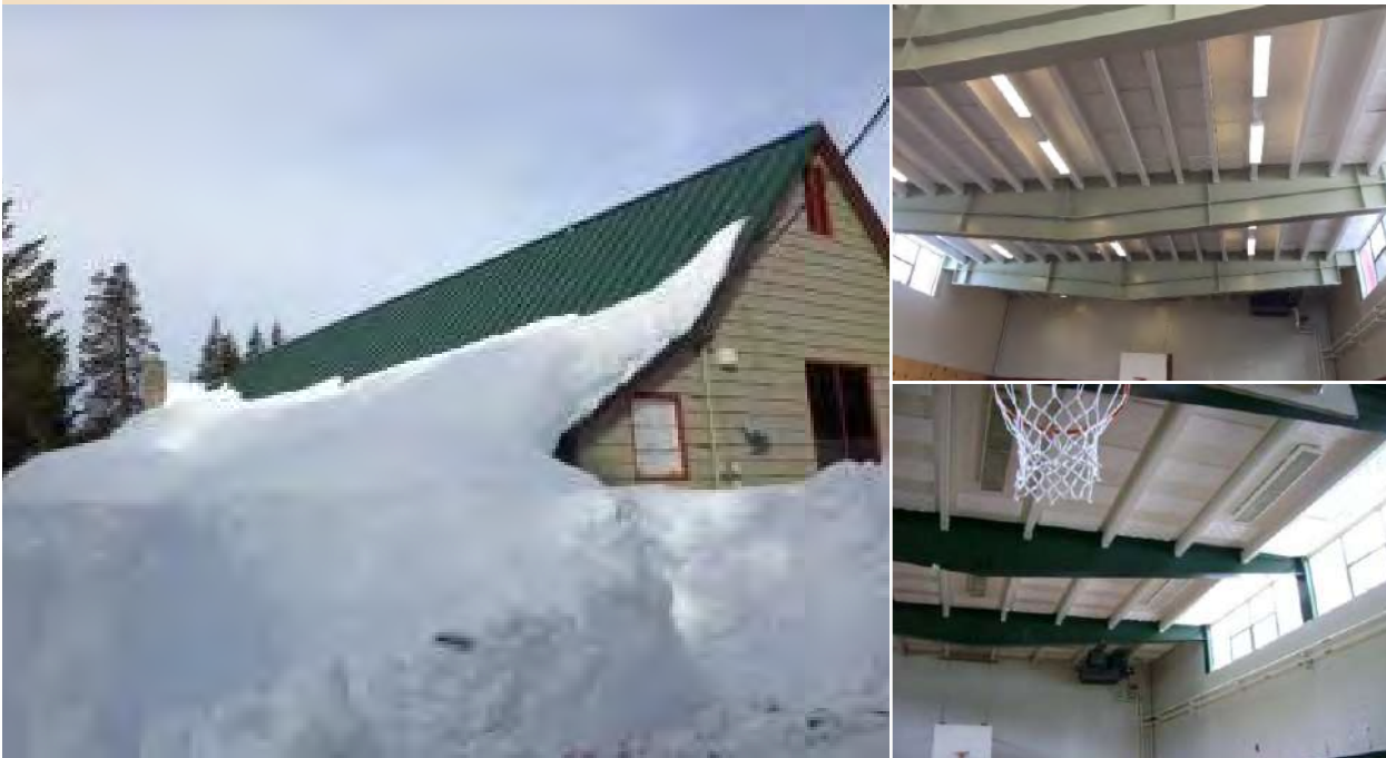
Clockwise from left: Donner Trail Elementary School from the outside; the interior of the roof before it was renovated to meet local building code specifications; the interior of the roof after it was renovated to meet building code requirements.
